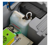
Chemical mixing system
